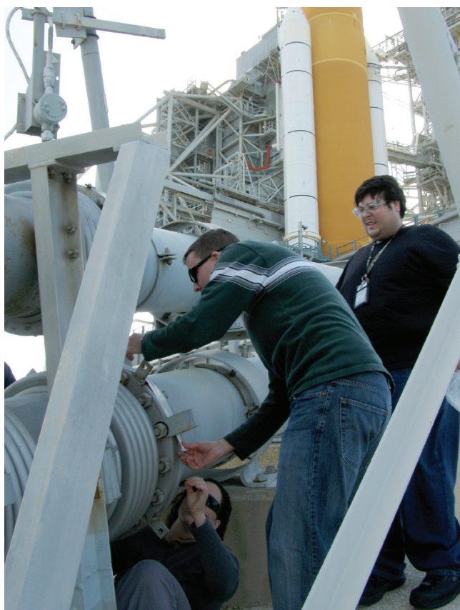
Robert DeVor (right) looks on while Luke Roberson and Angela Krenn apply hydrogen detection tape on a connector joint on a cross-country feed line. The piping connected the liquid hydrogen storage tank with the lines to fill the shuttle's external fuel tank on launch day.
