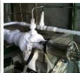
Cryo Test Main Fuel Valve
