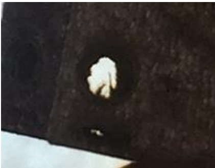
Needles due to excessive heat.
