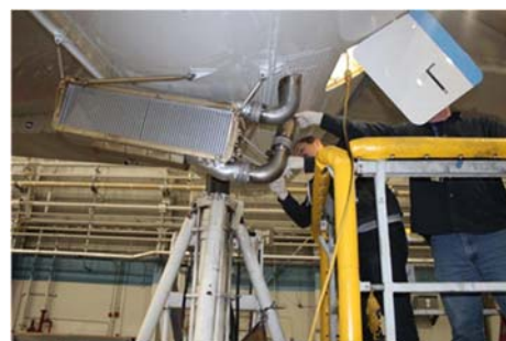
Figure 18 - Heat Exchanger Location on 757 (looking aft)
