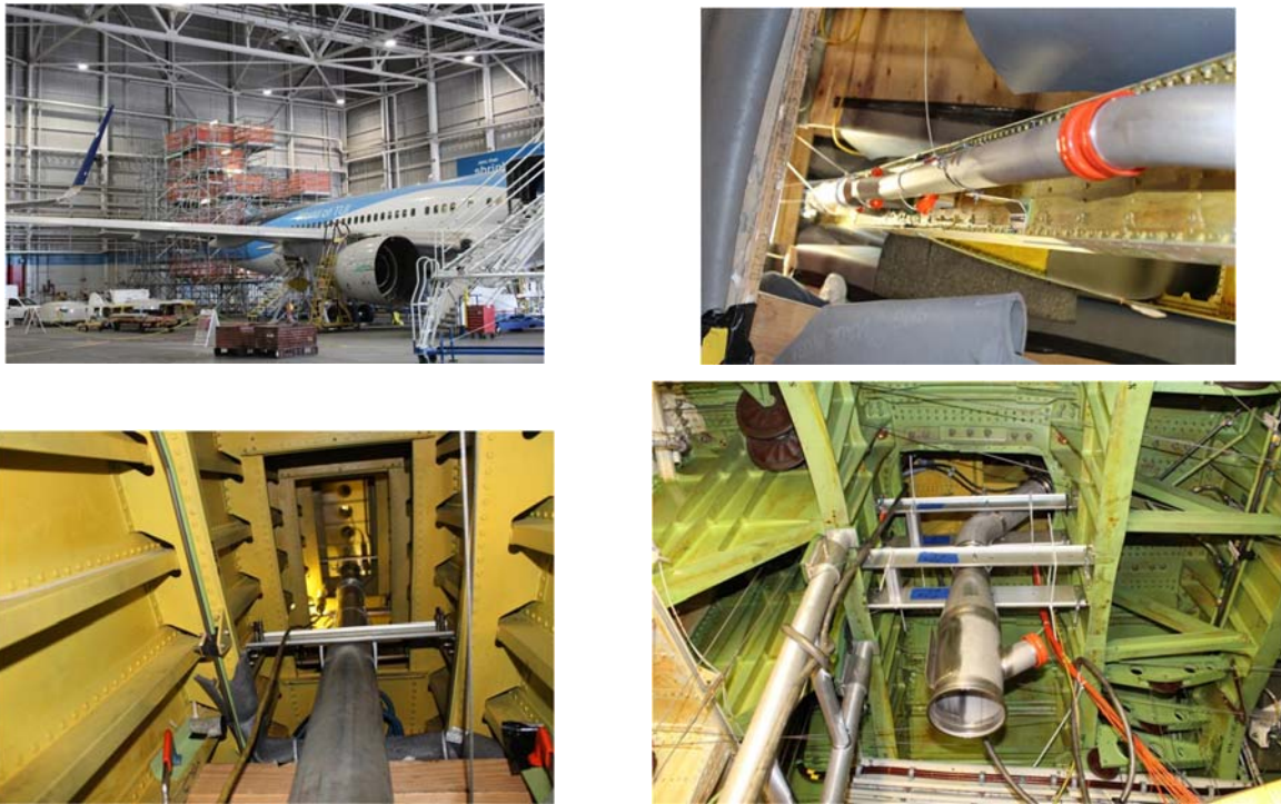
Figure 8 - AFC Ducting into the Vertical Tail
