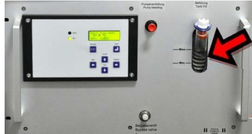
Figure 3-25: Water gauge on the SLR laser chiller
