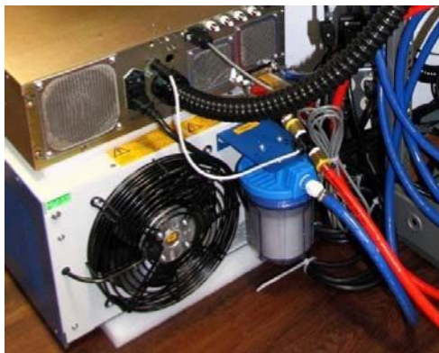
Figure 3-26: Coolant hoses for the Chiller and Controller
