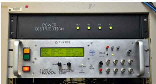
Figure 8-1: Power Distribution Box in Rack #2
