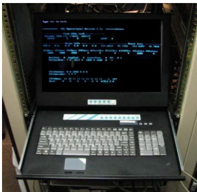
Figure 3-5: Rack mounted console
