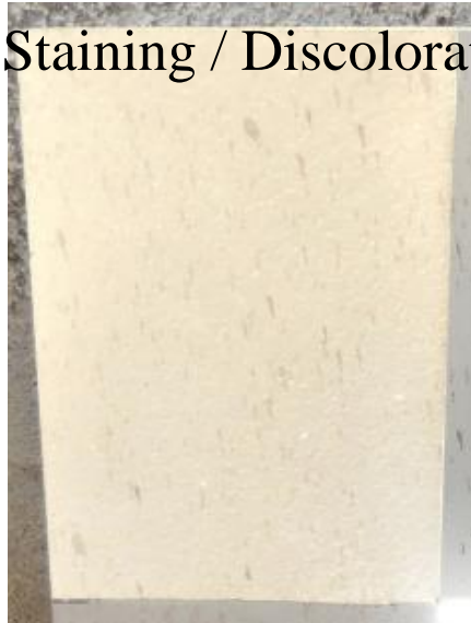
Exhaust Residue Adhered to Coating
