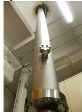
Cryogenic Container located at MSFC (below deck)
