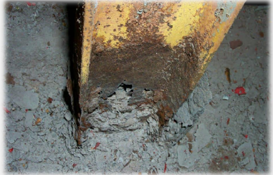
KSC Crawler/Transporter structural steel corrosion
