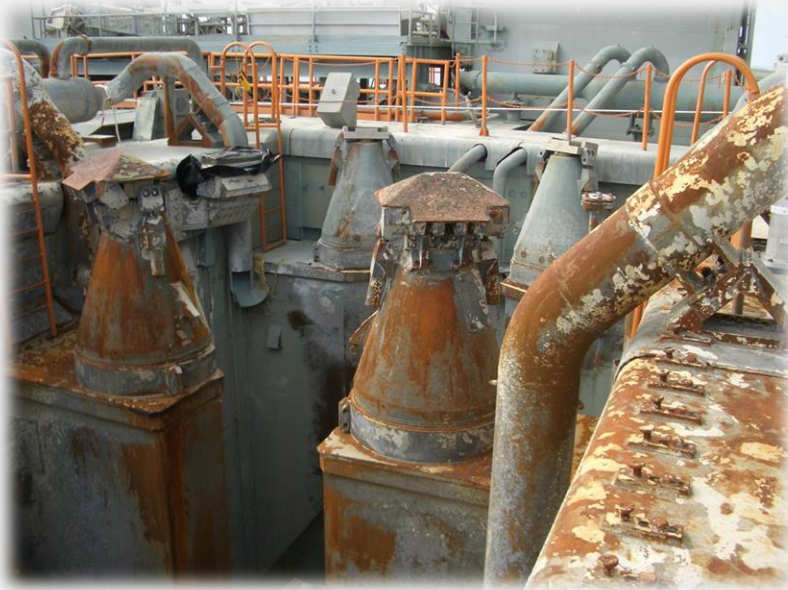
KSC Launch pad corrosion (after a Space Shuttle launch)
