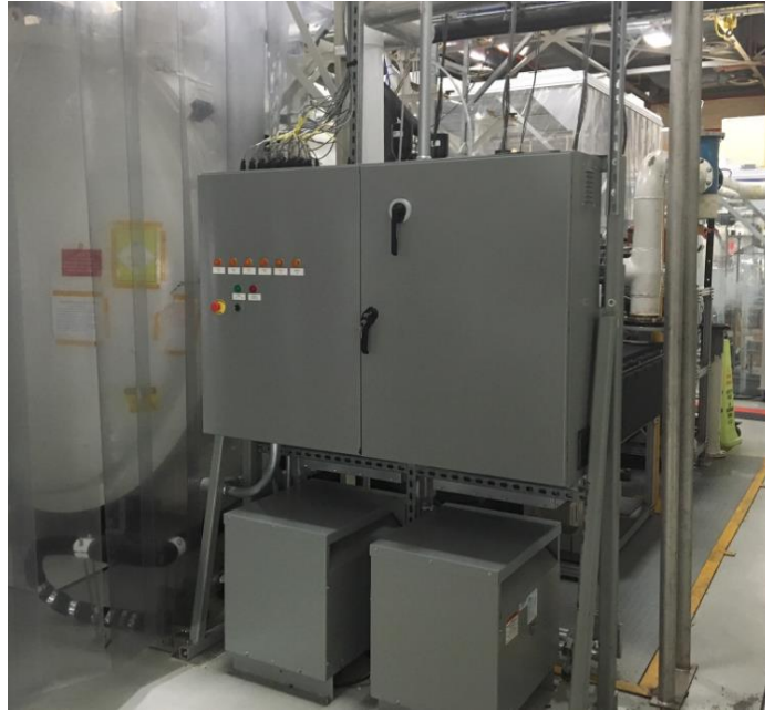
Figure 3 Heat Lamp Power Supply Enclosure
