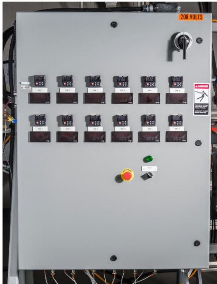
Figure 8 8x15 Auxiliary Heater Control System and Power Supplies
