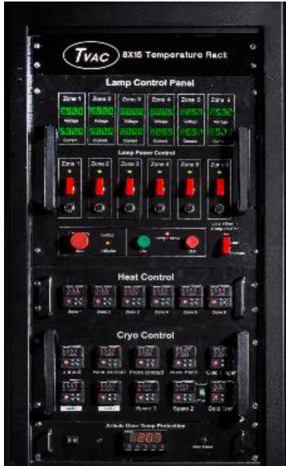
Figure 6 8x15 Temperature Control Panel
