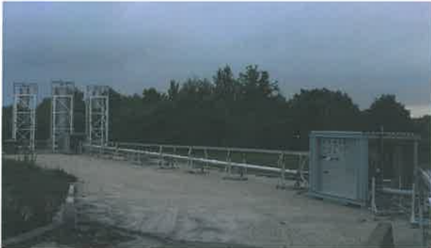
Figure 9. Valve Skids and Iron Rocket Tanks as part of the Autonomous Propellant Loading Test Site
