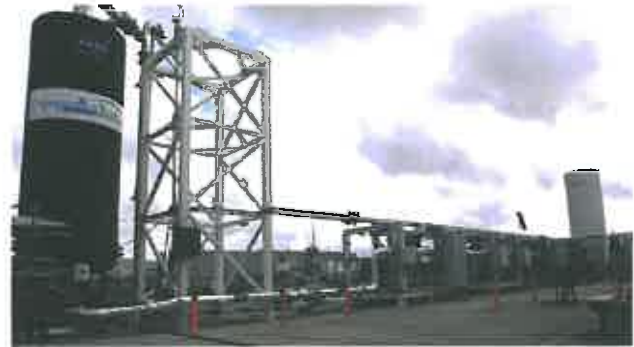
Figure 5. SPLS System at the KSC CTL
