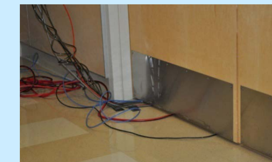
Typical cable run under chamber doors.
