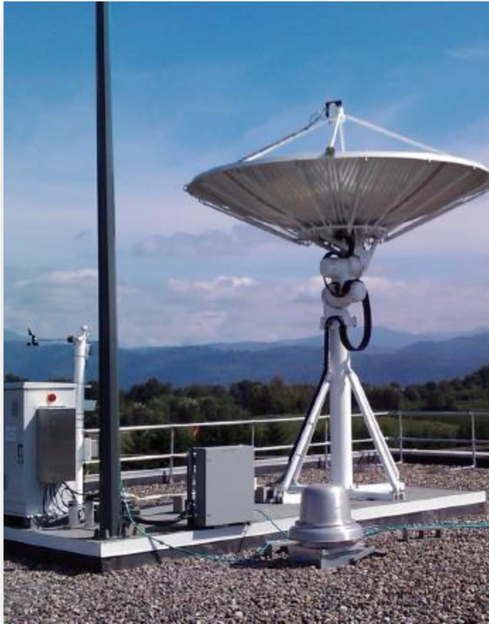
Type 2 Ground Mount on Roof
