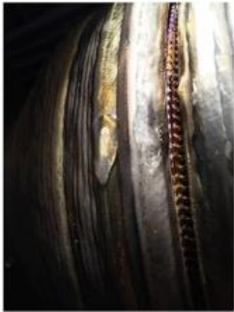
Before: Center Scaffold Opening ~1/8"
