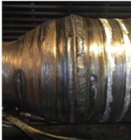
After: Hand TIG Weld Repair Completely Bridged All Gaps Around Center Scaffold
