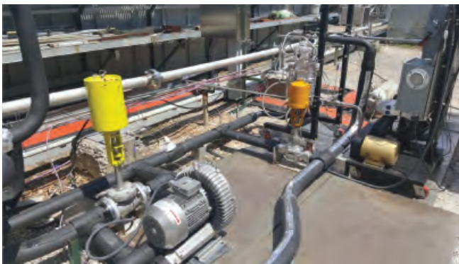
The blower and the heat exchanger loop are pictured above for the IVF "Phase B" testing.
