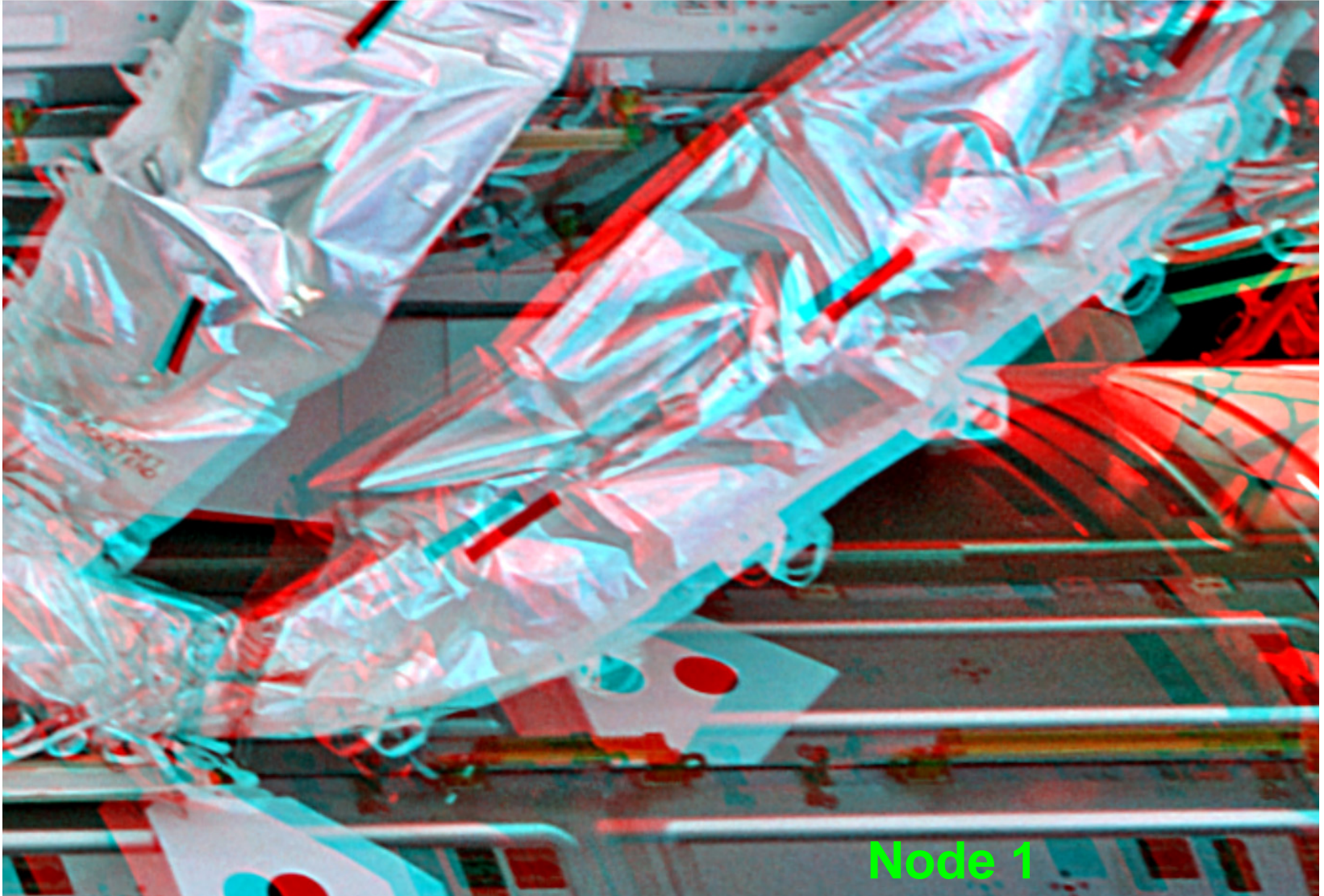
A closer view of the MLI wrapped ammonia lines.
