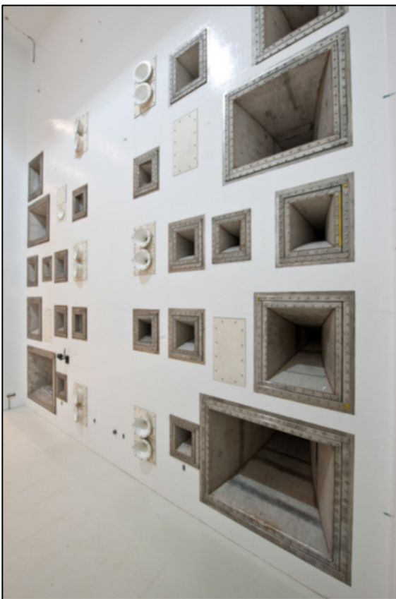
Figure 7.—RATF Horn Wall.
