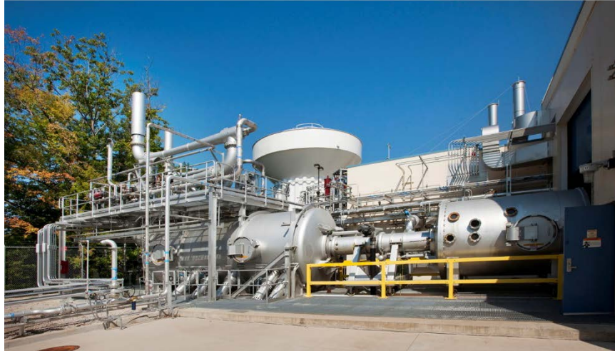
Figure 6: Photo of exterior of GRC Altitude Combustion Stand, showing ejectors, hydro-pillar, spray cart, water cooled diffuser, and mobile end of test capsule
