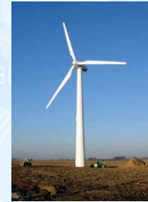
Wind Turbine Doubly Fed Machine
