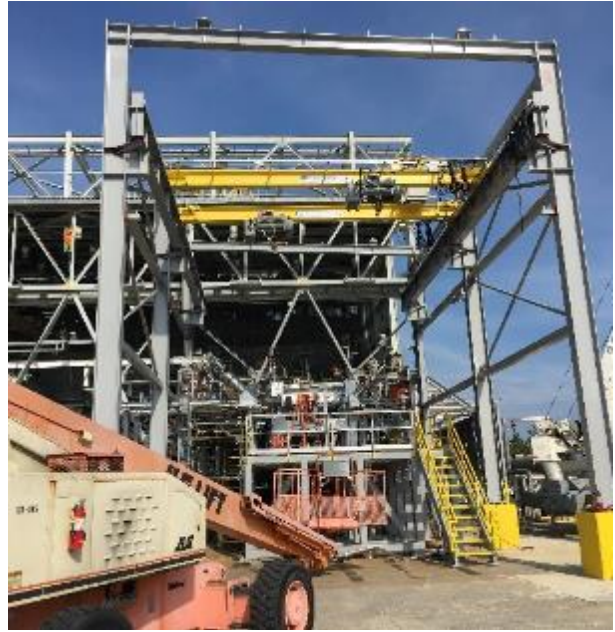
Fig. 38. Overhead crane structure being built at SSC Test Stand E1, Cell 1 for use with integrated testing.
