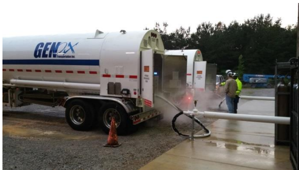
Fig. 28. LN 2 tankers connected to LN 2 fill system.
