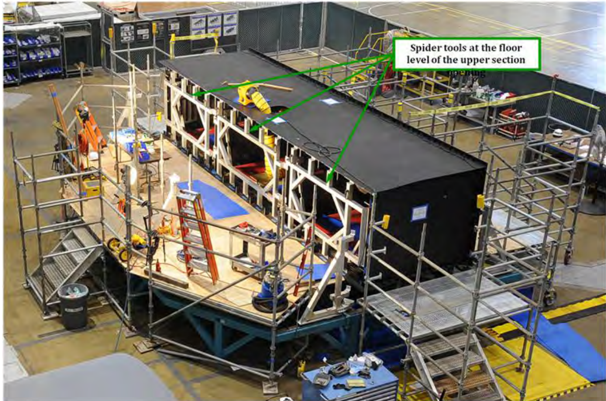
Figure 6-39. Upper Section With Spider Tools at the Floor Line of the MBB
