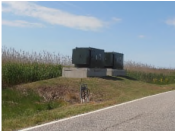
Figure 4- 44: Raised electricity utility boxes at Wallops Island. Photo taken by author June 2017.
