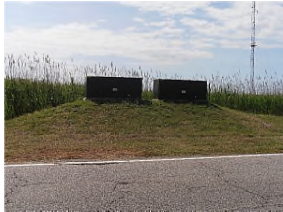
Figure 4- 43: Raised electricity utility boxes at Wallops Island. Photo taken by author June 2017.
