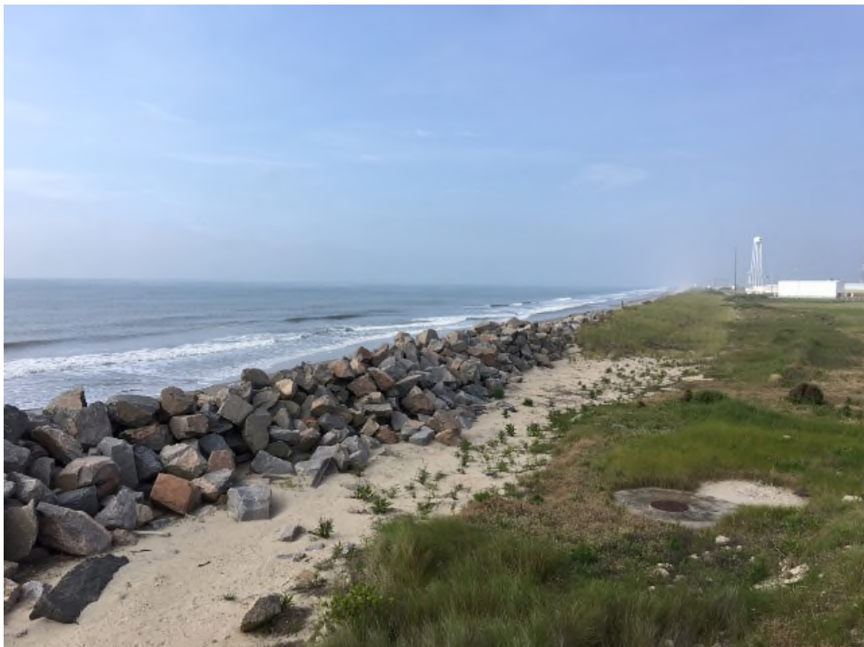
Figure 4- 7: Rock seawall at Wallops Island. Photo taken by author June 2017.
