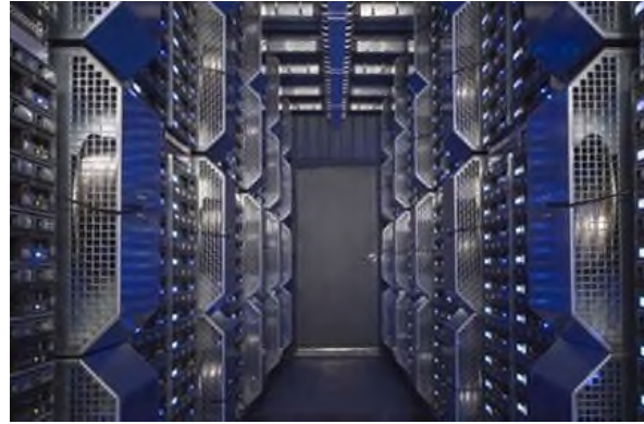
Figure 5- 7: Data Center inside shipping container. (The Royal Blog, 2008)
