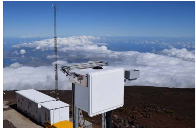
Figure 3. Installed Infrared Cloud Imager (7-11 um) with attached rain sensor
