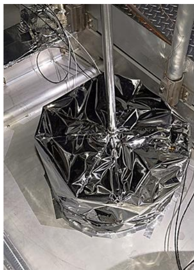
Figure 6. Down Rod Closeout
