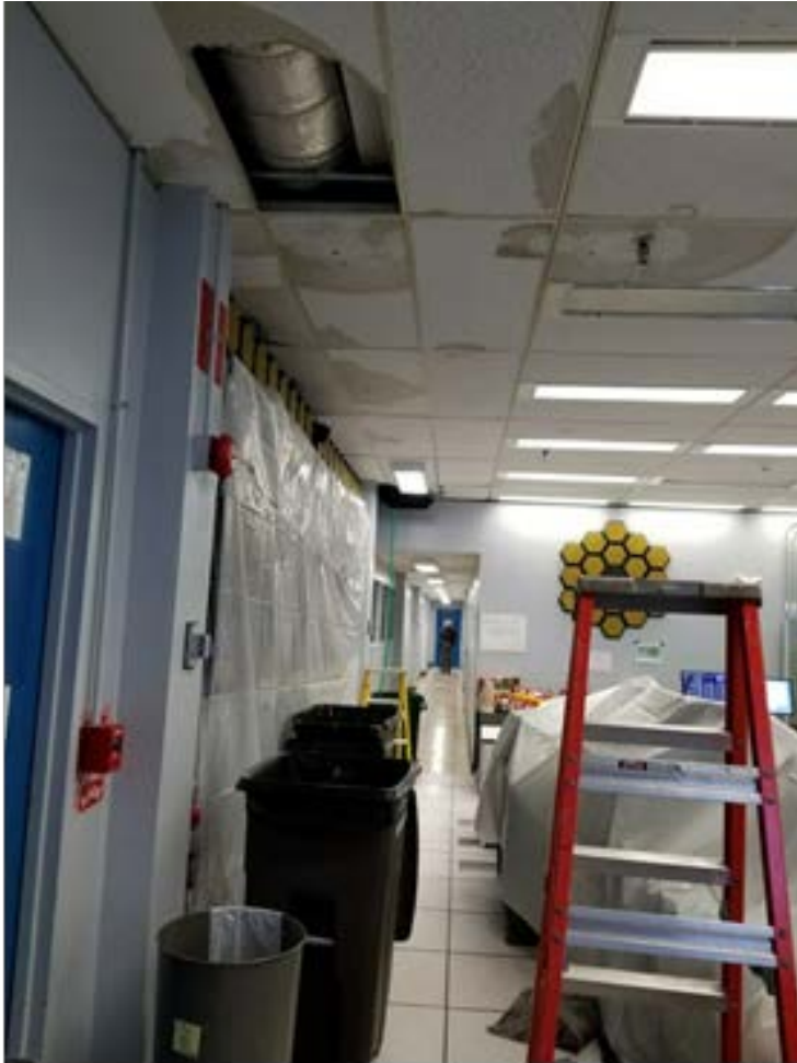
Water Damage in B32 OTIS Control Room, despite pre-test roof repairs
