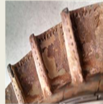
Typical build-up on blade
