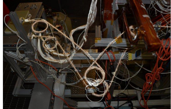
Figure 3. The propellant line coiled tubing wrapped in heat tapes for bakeout.
