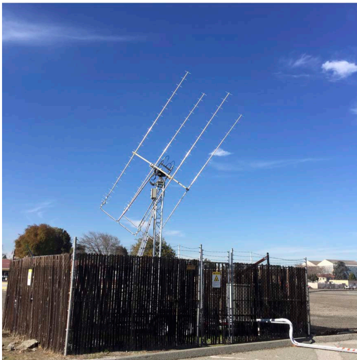
Figure 3-12— UHF Ground Station Mountain View
