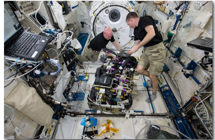
Carbon Dioxide Removal Assembly maintenance
