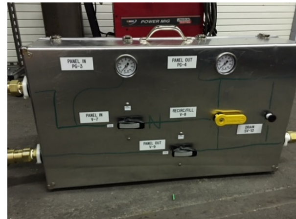
Figure 19: DI Water Portable Panel.
