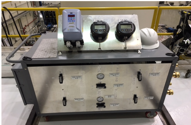
Figure 18: DI Water Fill and Drain Cart.
