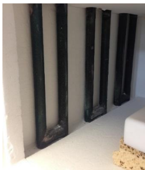
Figure 14. Cu deposition on furnace heating elements.
