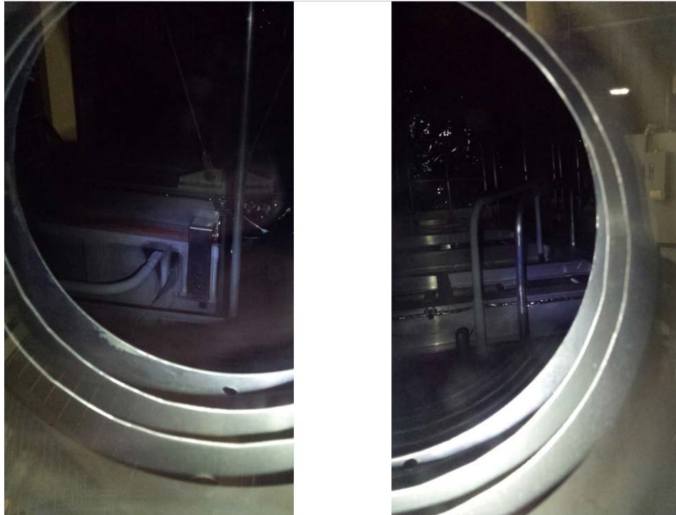
Figure 2: Visible Air Ice on Helium Shroud Piping
