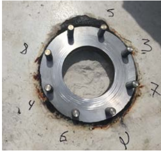
Figure 5, Field Machined Pearlite Fill Flange
