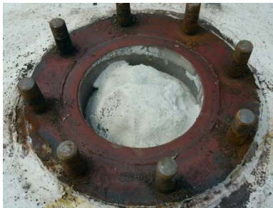
Figure 2, Pearlite Fill Flange Uncovered
