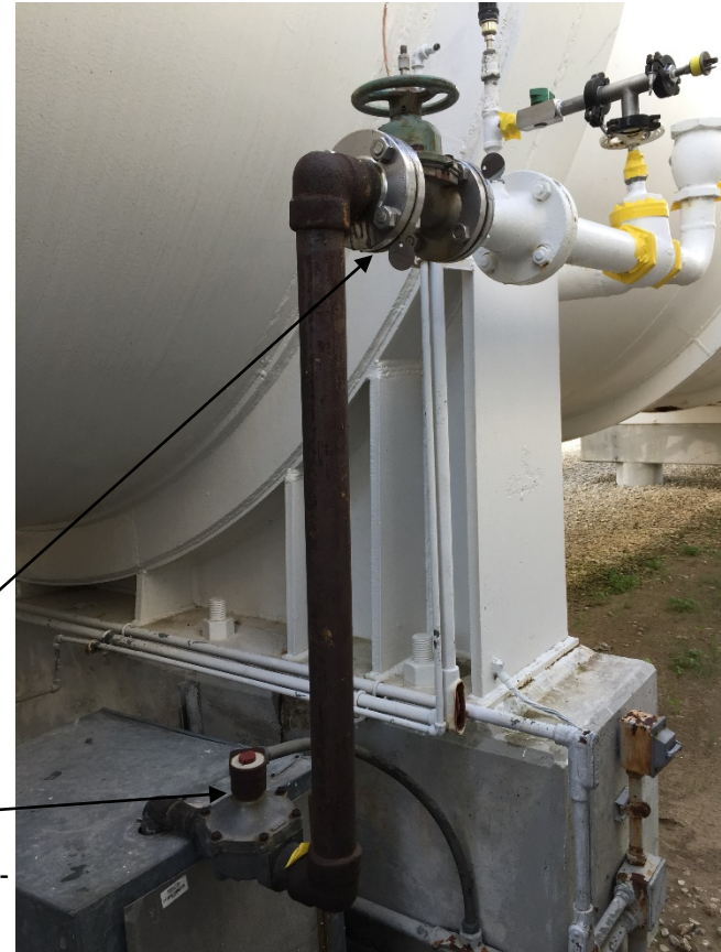
VACUUM PIPING WITH VALVE
