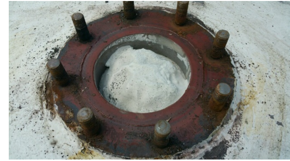
Pearlite flange with carbon steel flange.
