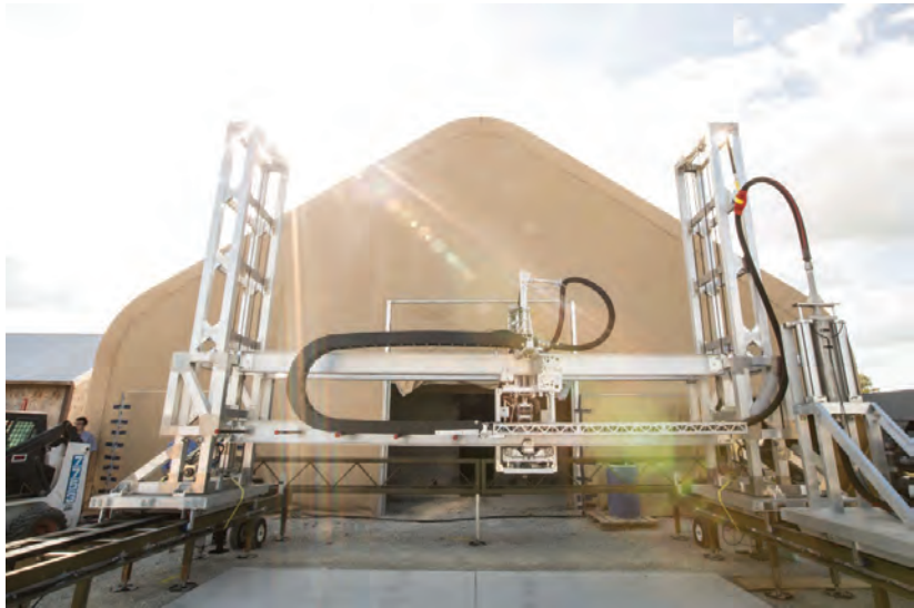
FIGURE 1. Through an Interagency Agreement, NASA and USACE are collaborating to advance the additive construction process. USACE's Automated Construction of Expeditionary Structures (ACES-3) gantry system will enable structures to be built within 1/8inch accuracy using six or less people in under 24 hr.
