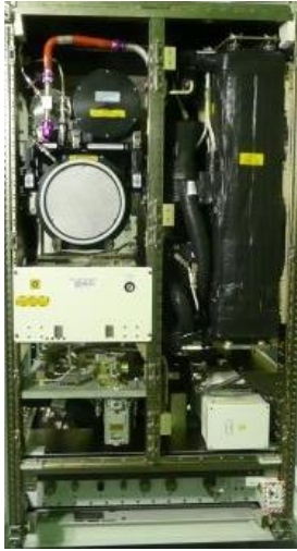
Atmosphere Revitalization System Rack (Activated Feb 2001)
