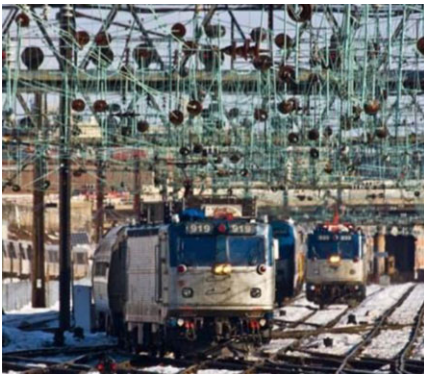
Figure 8.6. Northeast Corridor catenary & power supply systems. Source: http://www.nec-commission.com/cin_projects/catenary-power-supply-systems/ .
