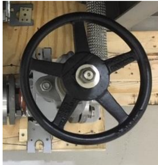
Figure 15. Overhead of Manual Valve Mount. Image Credit: Giovanni Campos, NIFS Intern.
