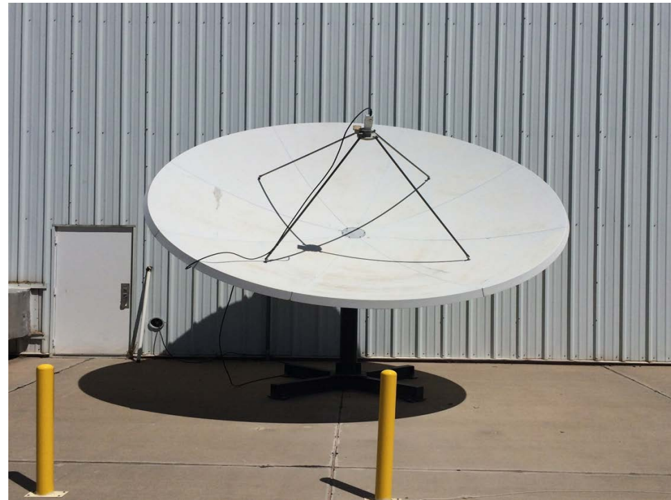
NOAAport Installation in Fort Sumner, NM
