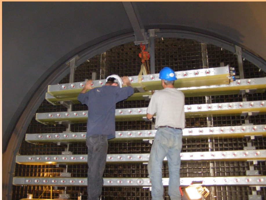
18-ft Plenum and Spraybars
