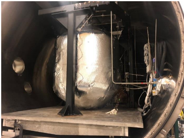
CryoFILL Liquefaction and Storage
