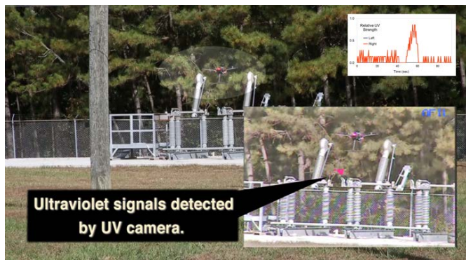
Figure 2. Validation of the compact UV sensor signal with corona camera in a substation measurement flight. The visible camera image shows the UAV above the substation structure (background; UAV is in lightened ellipse). The inset at top right shows the compact UV sensor recording, which reaches a maximum as the UAV passes the corona generator. The inset at bottom right shows the corona camera record; the bright red blobs at the center of the image are locations of UV emission.
