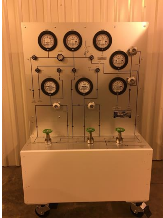
Figure 2. Methane Servicing Panel
