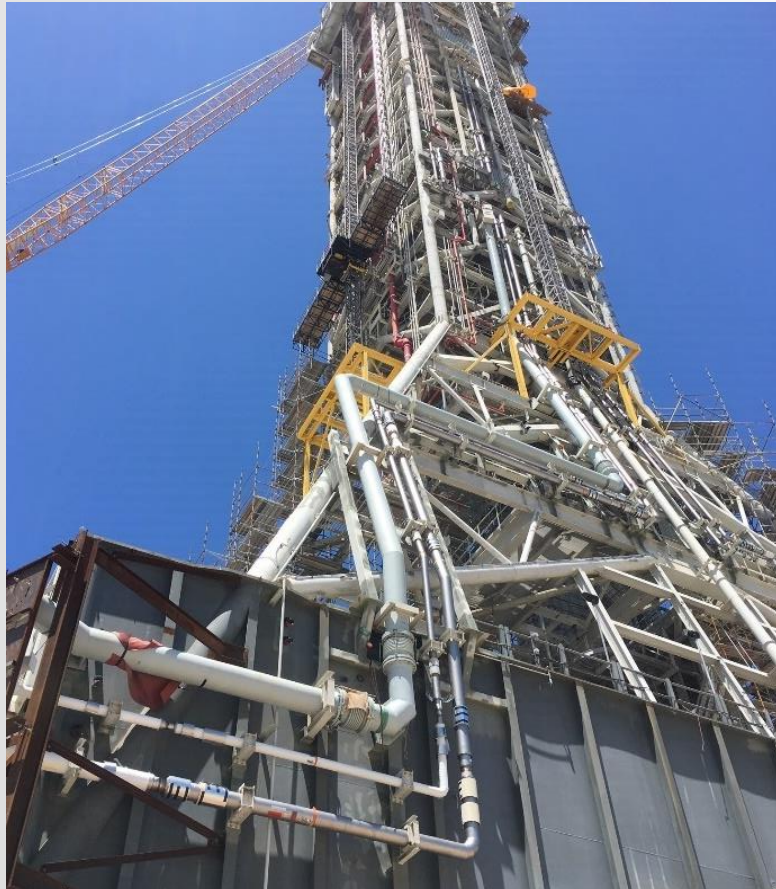
Transfer piping: normal vacuum ( \sim 1\mu )
