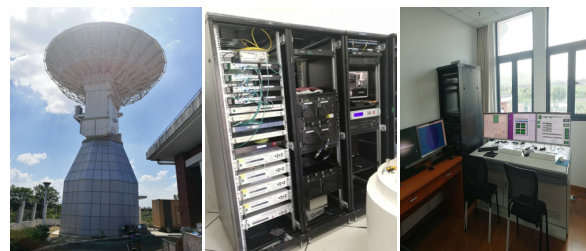
Fig. 1 The TmVGOS antenna (left), VLBI terminals (middle), and observation room (right).
