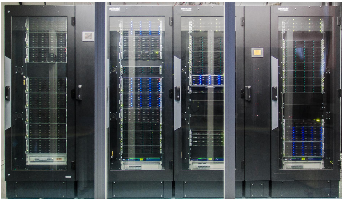
Fig. 1 New HPC cluster at MPIfR seen through a glass wall.
