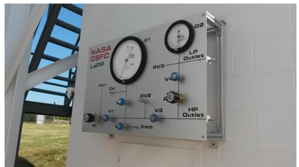
Figure 8 Pressure Control Panel
