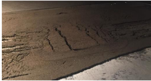
Figure 7. Composite feed bed cracking due to high heat
