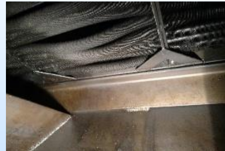
Heat Exchangers Tube Modules Damaged and Removed for Repair
