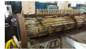
Support for the LaRC Compressor Station Heat Exchanger Repair Keeps Facilities Running
