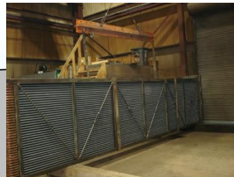
Heat Exchanger Module Checks
