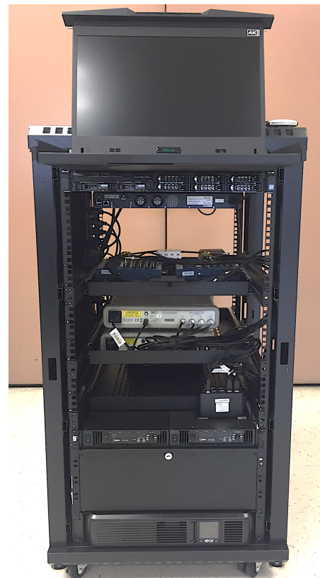
Figure 13. OCI Limited Performance Test EGSE Rack
