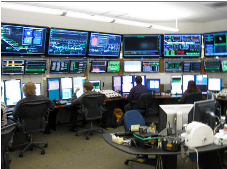
Figure 20. PACE Control Room
