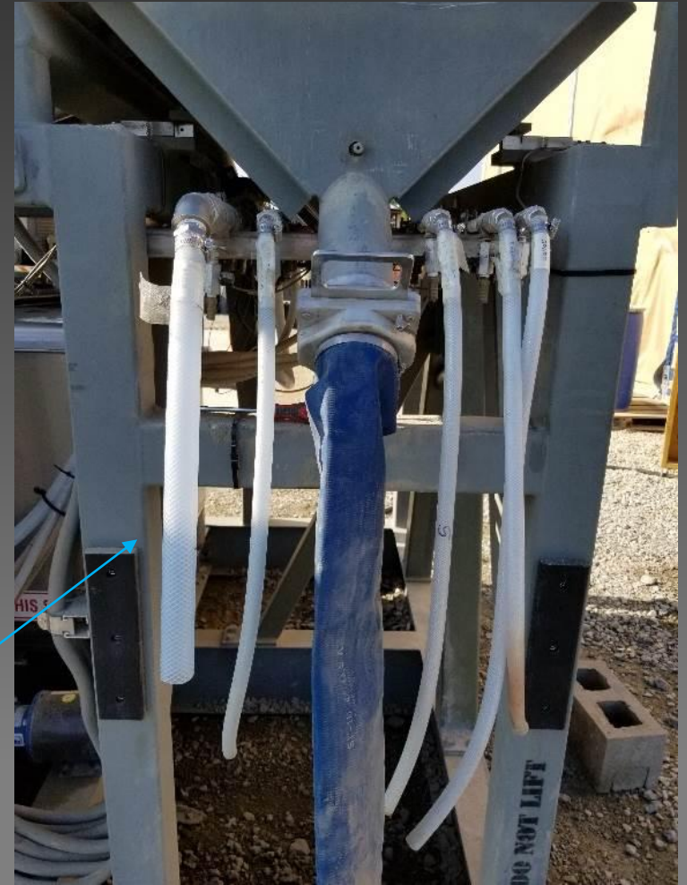
5 Liquid Discharge Pipes
