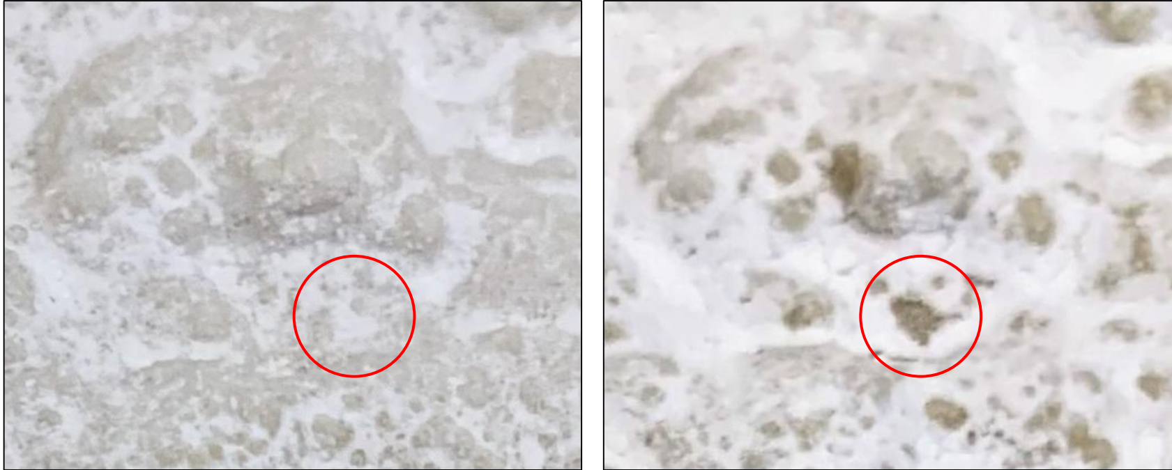
Potential Issue with Coating Flaking Off When Too Thick
